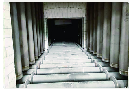
Furnace rollers in use
